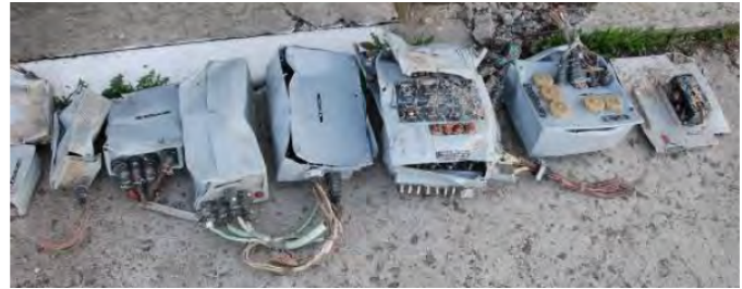
Figure 1.17: Junction and control boxes of electrical installation. Photo taken at the site of wreckage storage [16].
